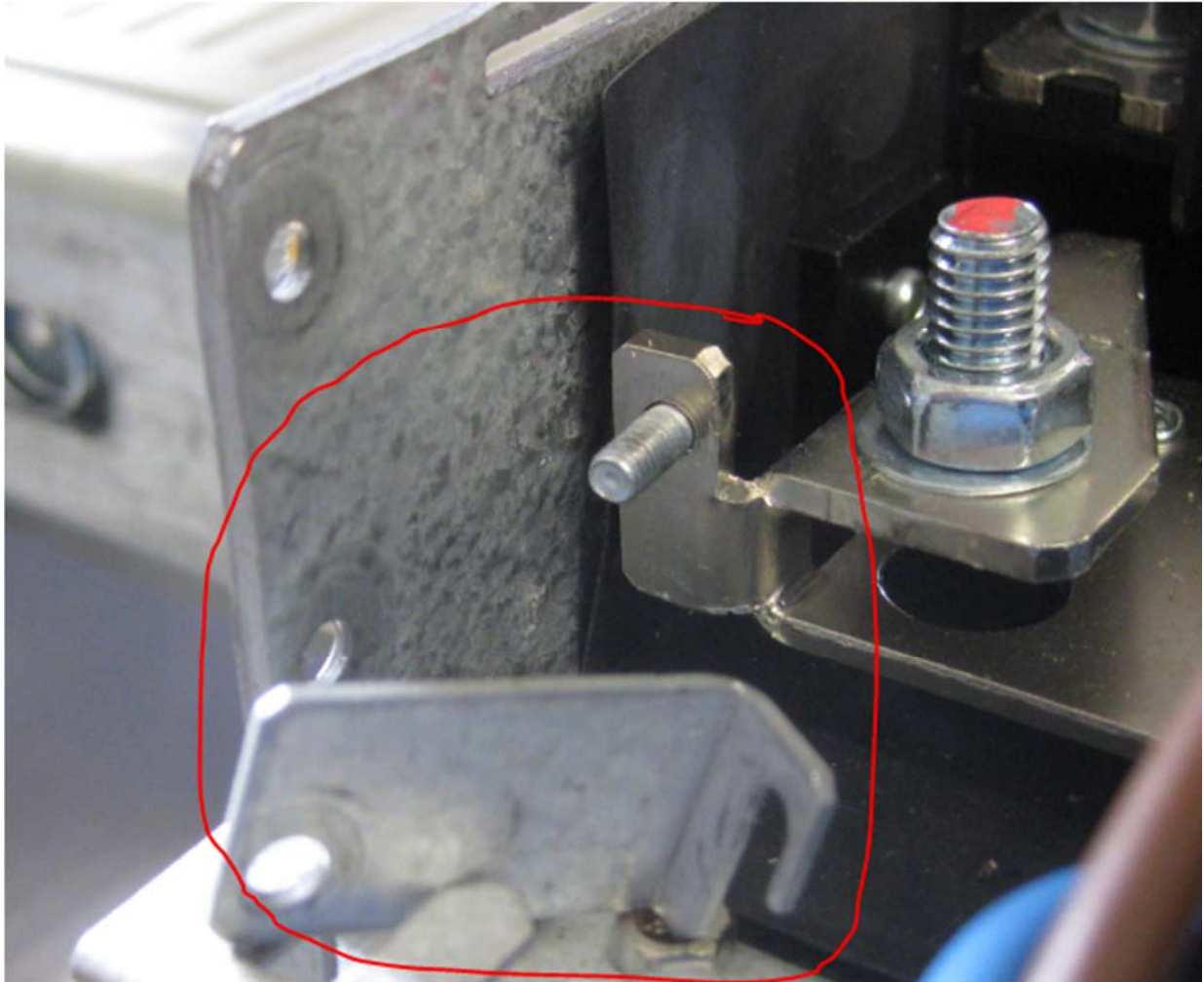
Figure 20. Chassis & DC Negative Earth
